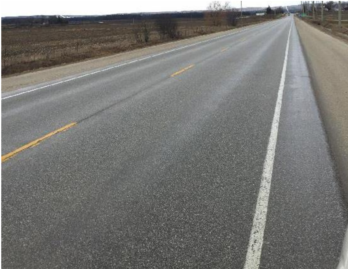
Figure 3. Excellent pavement condition seen in a road which had been recycled using CIR 14 years prior (Highway 91, Simcoe County, Ontario).
